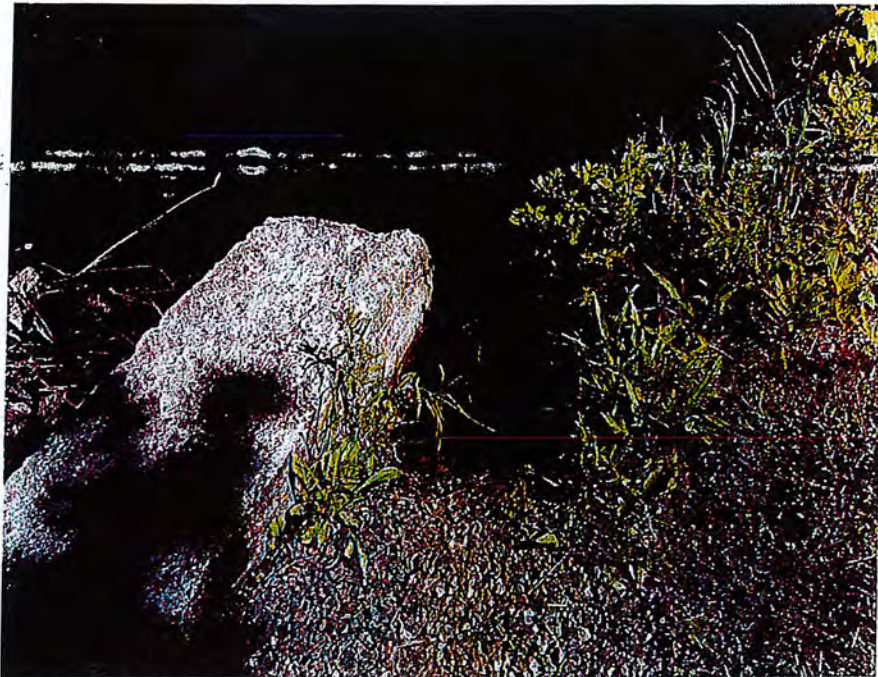
Photo 17: Deficiency – Scour at upstream slope
