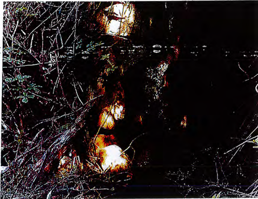
Photo 19: Deficiency – Leakage behind the left training wall
