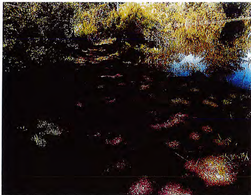
Photo 22: Deficiency – Bare soil and low area at the middle of the dam
