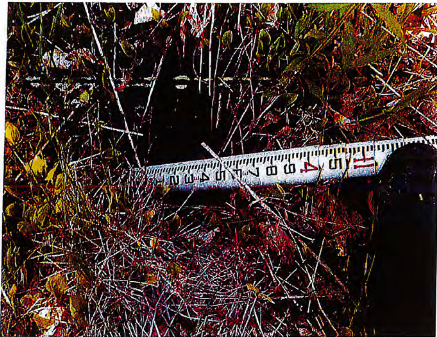
Photo 21: Deficiency – Animal burrow on the right abutment
