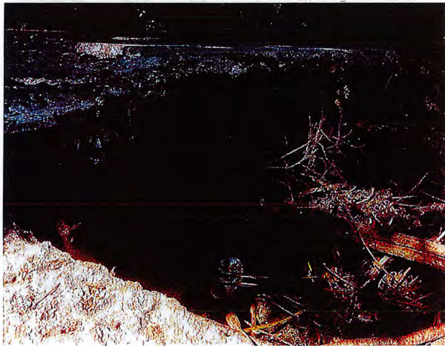
Photo 18: Deficiency – Debris blockage at the approach to the spillway
