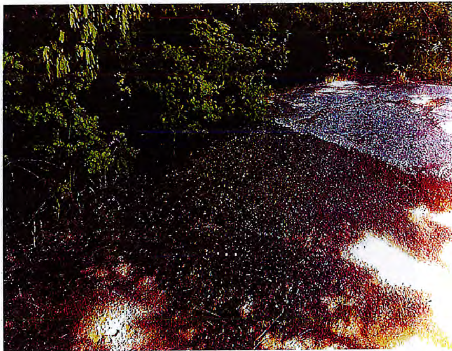
Photo 20: Deficiency – Settlement and area of crushed stone placed at the left side of the spillway
